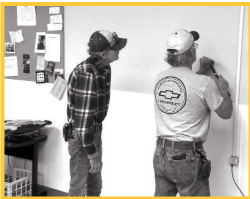
Staff members Lonnie Callies (left) and Larry Moeller prepping the wall to put up the smartboard frame.
